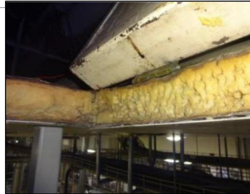
Expanded polyurethane = Combustible (slow burning)
